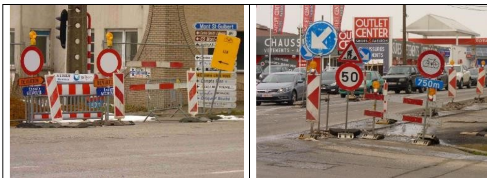
Figure 46: insufficient alternative cycle infrastructure during road works © Transport & Mobility Leuven
