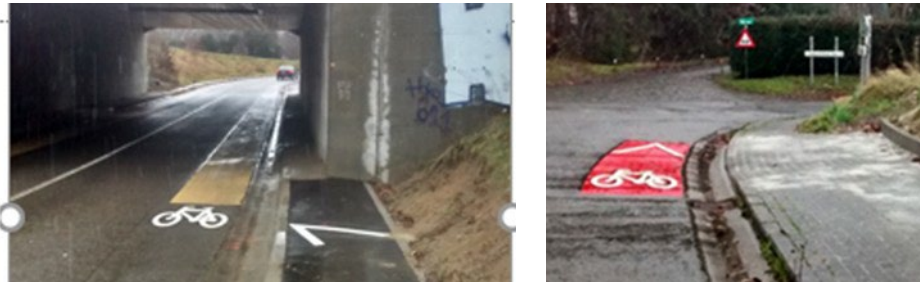
Figure 40: cycle path arranged over 100m with unsafe cycle path ending © Transport & Mobility Leuven
